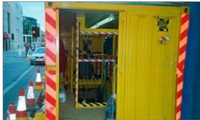
Figure 12 - HV cable jointing container
